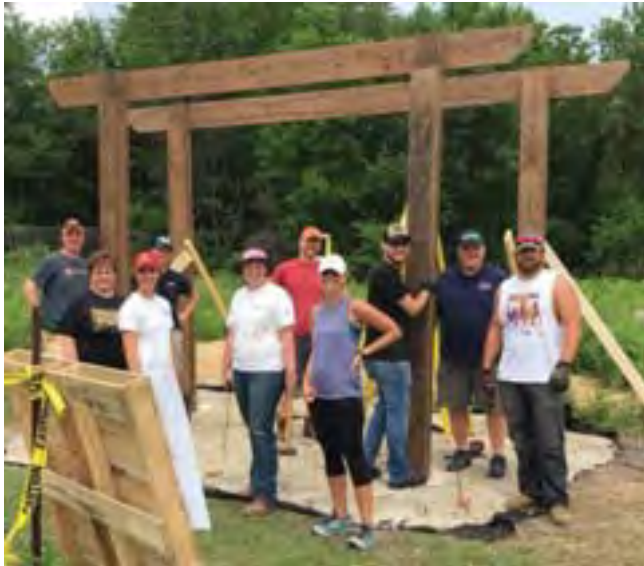
Members of the Iowa Valley Leadership Class of 2018 working on the pergola at GrimesFarm.
